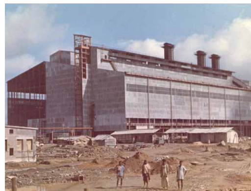
The LD steelworks in Rourkela, India during the construction phase (Photo: Steel History Club).
