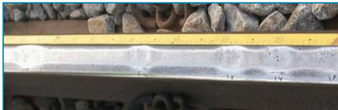
Squats: V-shaped or half-moon-shaped hollows, especially from heavy haul traffic. Tears are growing beneath the surface
